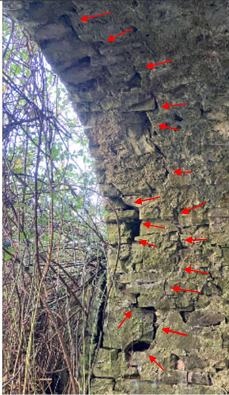
A1. Cracking, separation of arch ring, left arch
