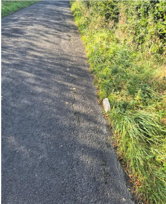
Figure 3 - Collapse of road along western edge
