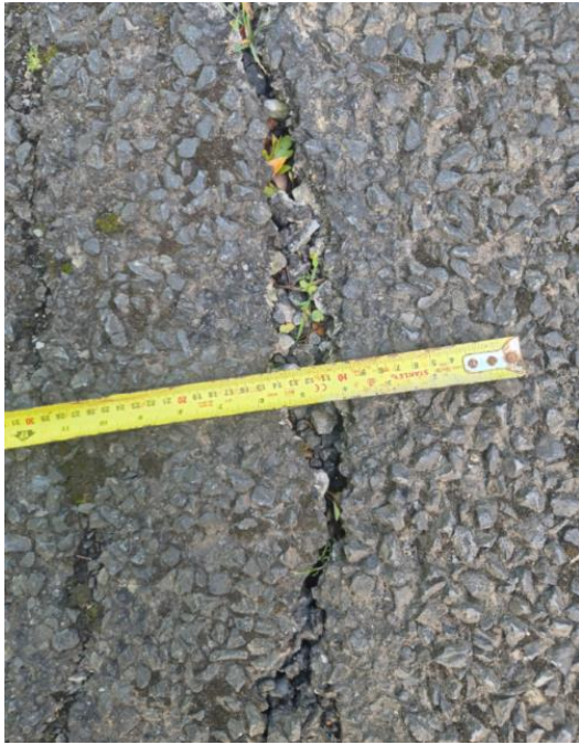
Figure 8 - Cracking along crown of road
