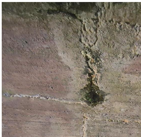
Figure 19 - Hole in concrete lining
