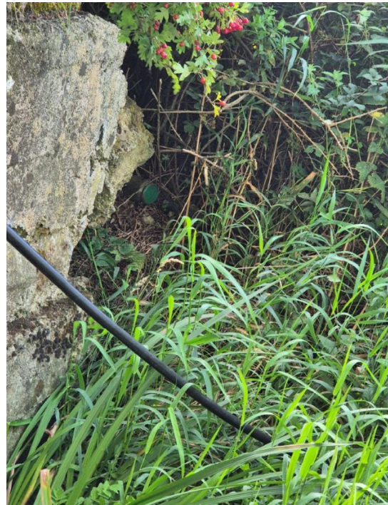
Figure 6 - loss of ground to culvert approach wall
