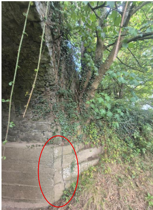
Figure 14 – Cracking of scour works
