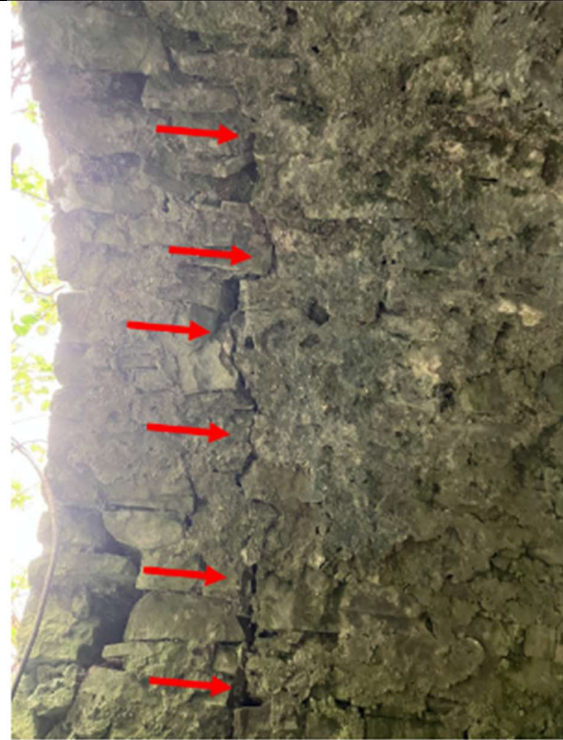
A2. Cracking, separation of arch ring (close up)
