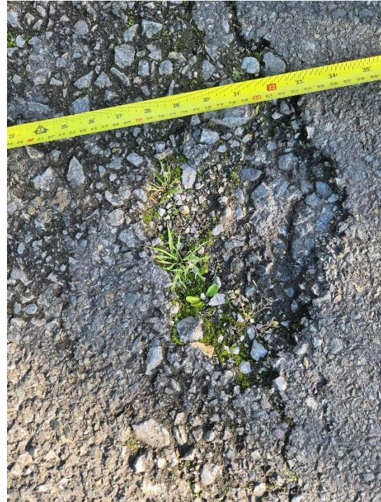
Figure 4 - Unravelling of road surface
