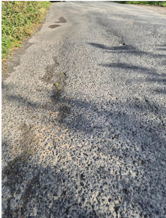
Figure 5 - Settlement of road on southern approach to culvert
