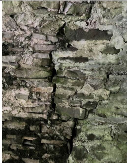
B2. Bulging and radial displacement, left arch barrel
