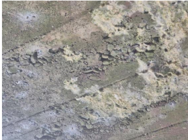
Figure 18 - Concrete lining degradation
